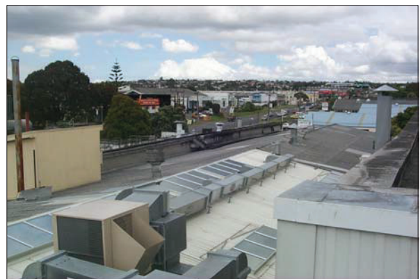
Typical Roof-Mounted HVAC
