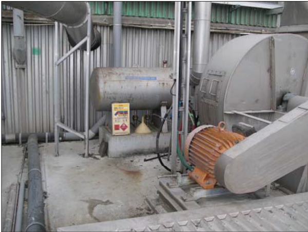
Motors and Bearings are Everywhere – and so is Fuel for Fire
